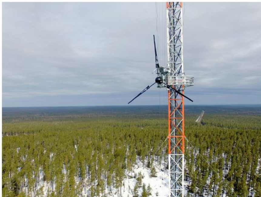
Windular's state-of-the-art hybrid wind and solar systems on Bell's Nungesser Lake tower site in Ontario.
